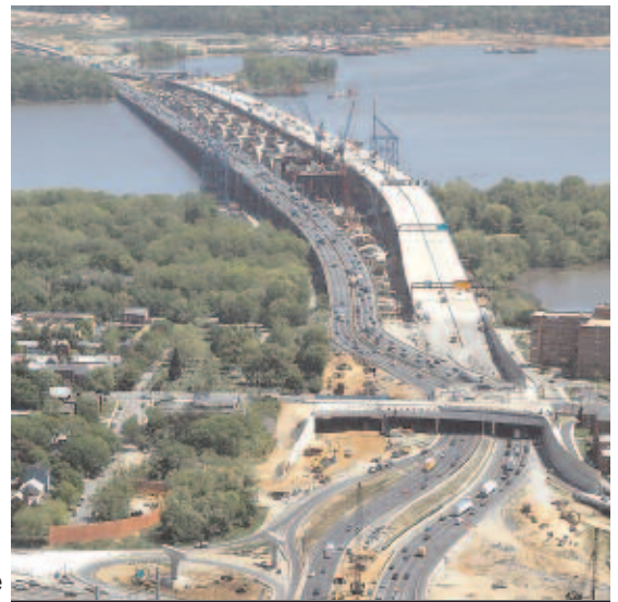
Woodrow Wilson Bridge Replacement Project, looking North from Virginia side (foreground) to Maryland side. Demo took place in lower left corner area.
